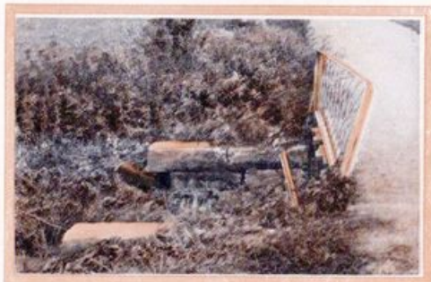
This is where the car ran into the bridge-abutment at forty-miles-an-hour. Notice the stone pushed out of place
